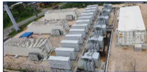
Hagåtña 24 MW Energy Storage Batteries
