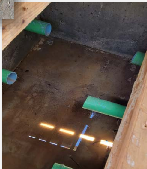
Inside of lifting station
