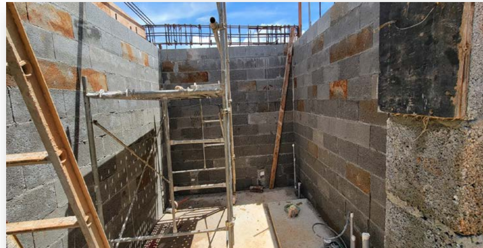
Inside of Electrical Room
